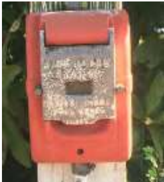
Current Pull Box for Emergency Assistance (3 rounds of 5 blast)
