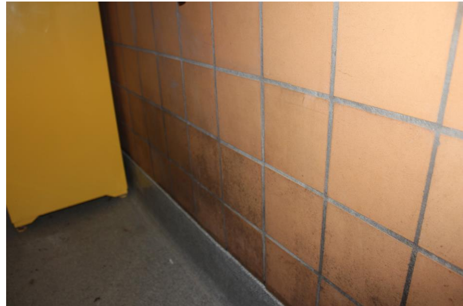
Exhaust particulates cover every surface within the station, causing an extremely unsafe condition
